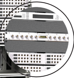
Power Supply Distribution boards
